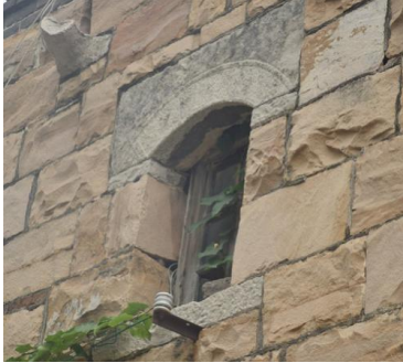
Fig. 5 Jining - Wudai Mountain Village: The window linings are made of three pieces of stone with a width of about 120mm. Seen from the front facade, it looks very atmospheric. The lintel has an arc pattern.
