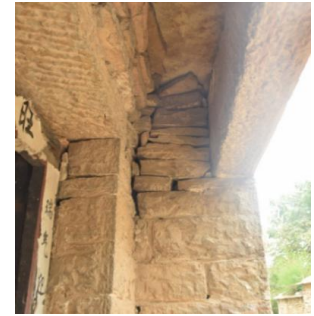
Fig.7 Taian-Chaoyang Zhuang: The door lintel has an independent riding stone outside and an independent door lintel inside.
