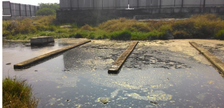
Fig. 3 Unscientific leachate pond at UD landfill, Pune, India
