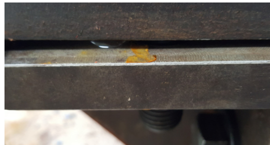
Fig. 7. Leakage at straight line
