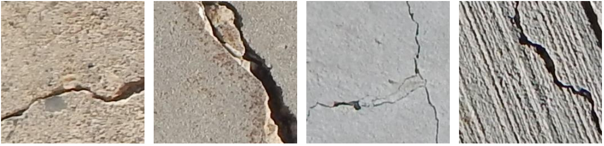
Fig. 1. Concrete crack images from USU
