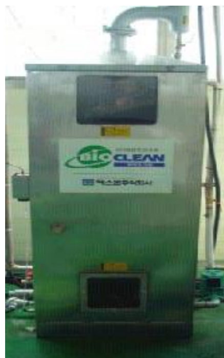
Figure 3: The View of VOCs Control System with Biofiltration
