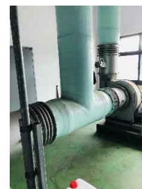
Figure 8: Branch duct of pipe
