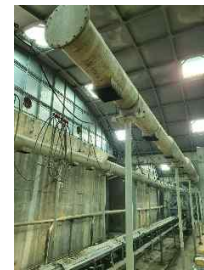
Figure 6: Hood odor trap
